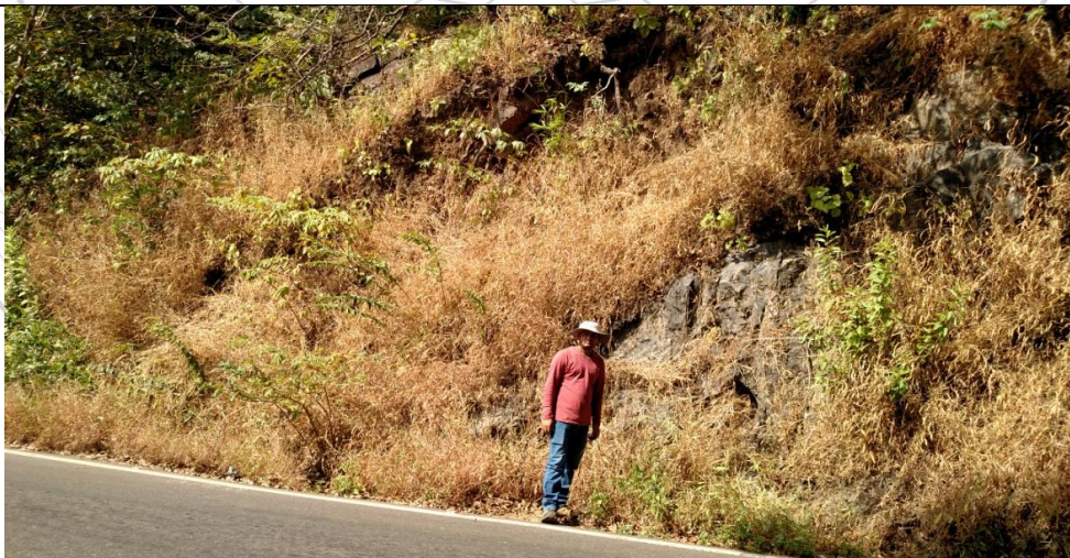
Photo3: Field Photographs showing Extensive Cut Slope along Anmod-mollem Ghat road NH-4A
